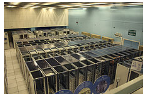
The CERN data centre in 2010 housing some WWW servers
